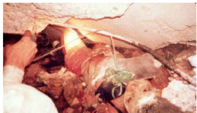
Figure 6:4 Collapse on a Victim
